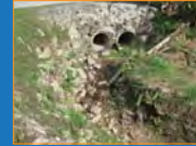
Assumption Drive, Pitti - May need culvert structure.
