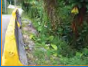
Ocean Summit Drive, Pitti - Safety issues with steep shoulder drop-offs.
