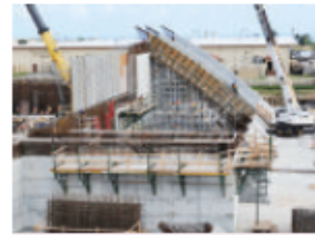
MILITARY CONSTRUCTION: Photo shows construction on the Pacific Air Power Resiliency Tanker Group Maintenance Hangar project on Andersen Air Force Base on Feb. 27, 2019. The Navy this week awarded another $43 million project to be constructed on Andersen by local contractor Core Tech-Hawaiian Dredging. Photo courtesy of U.S. Navy
